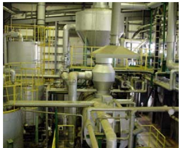
Photo. Equipment for food waste recycling
