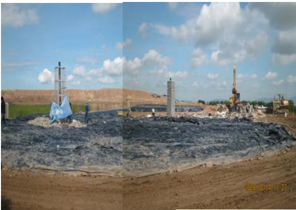
Photo: Construction of test cells at Laem Chabang landfill. The black sheet covering the surface is an alternative to daily soil covering to prevent an indescribable odor and many, many, many flies.
