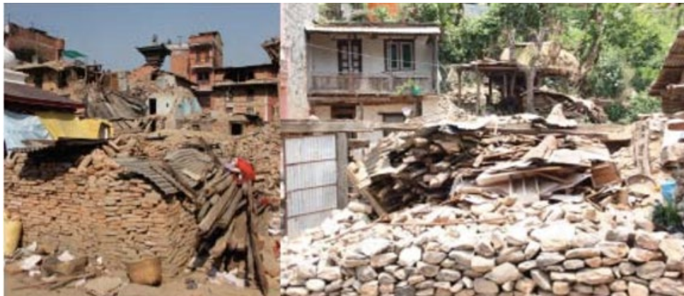
Figure 10 Segregation of recyclable objectives (Bricks, Stone, Wood, Iron, Roof tin sheet, etc.) from disaster wastes
